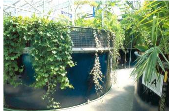
Living machine wastewater treatment
